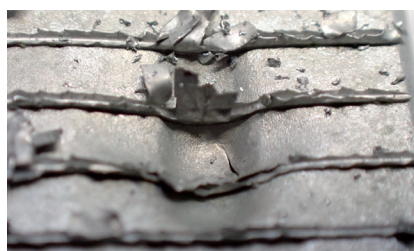
Figure 2: Deformation due to ice droplets on the evaporator pipe
